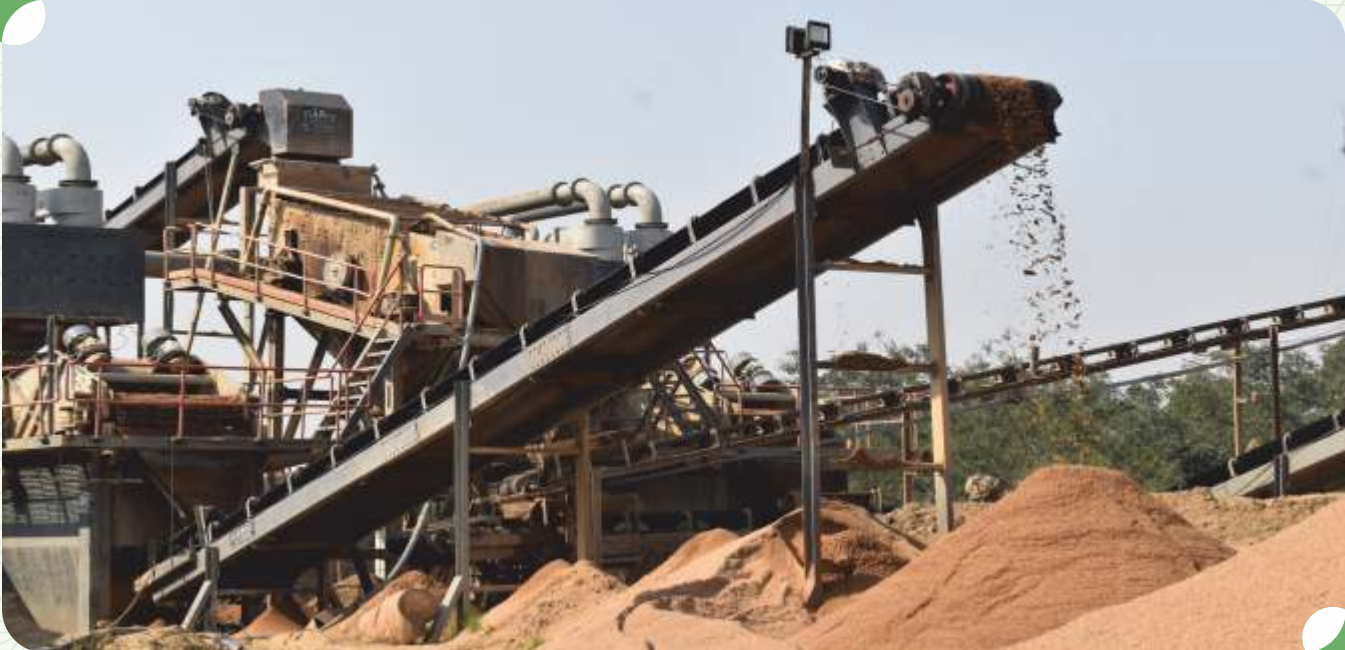
■ Sand Segregation Plant in operation.
