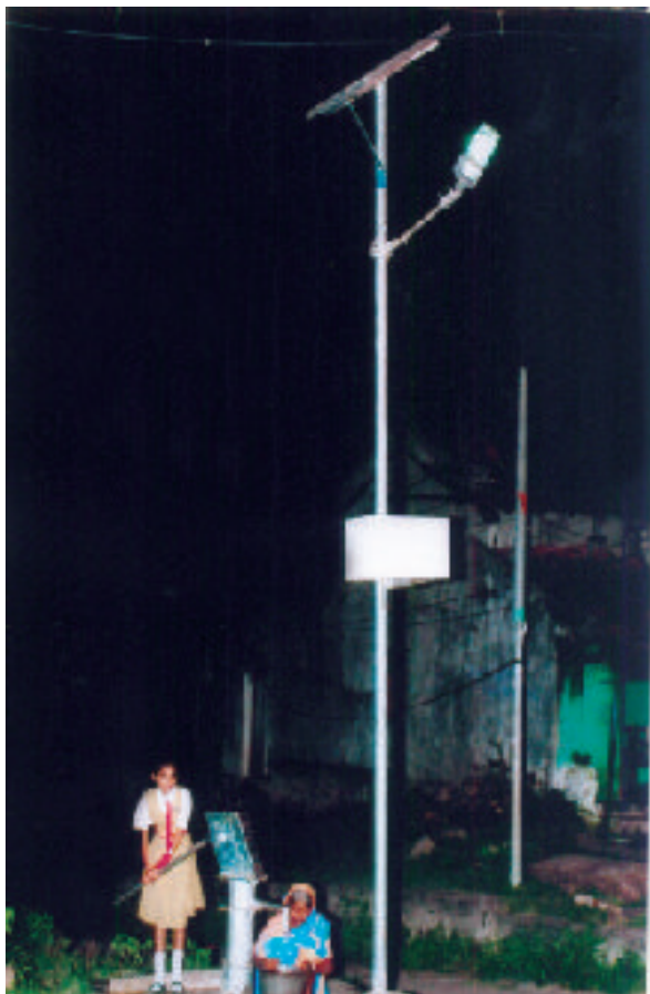
A CSR Gesture - Water hand pump and solar street lamps were installed in a village near one of the mine of WCL
