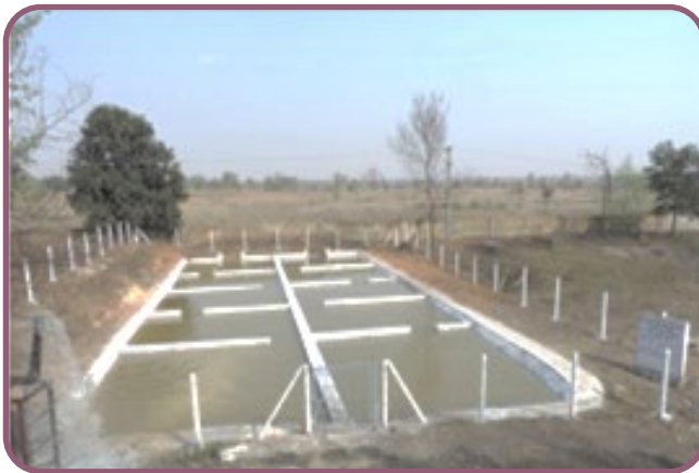
Settling tank for treatment of Mine Water, Rehar UG
