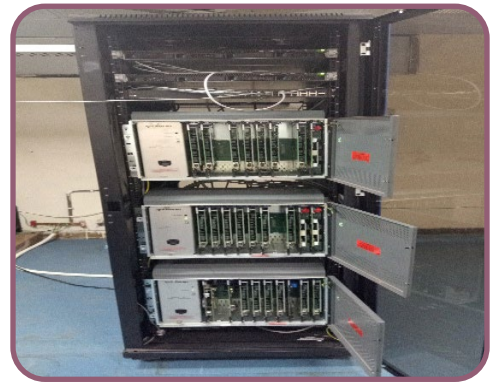
IP based Telephone Exchange at SECL HQ
