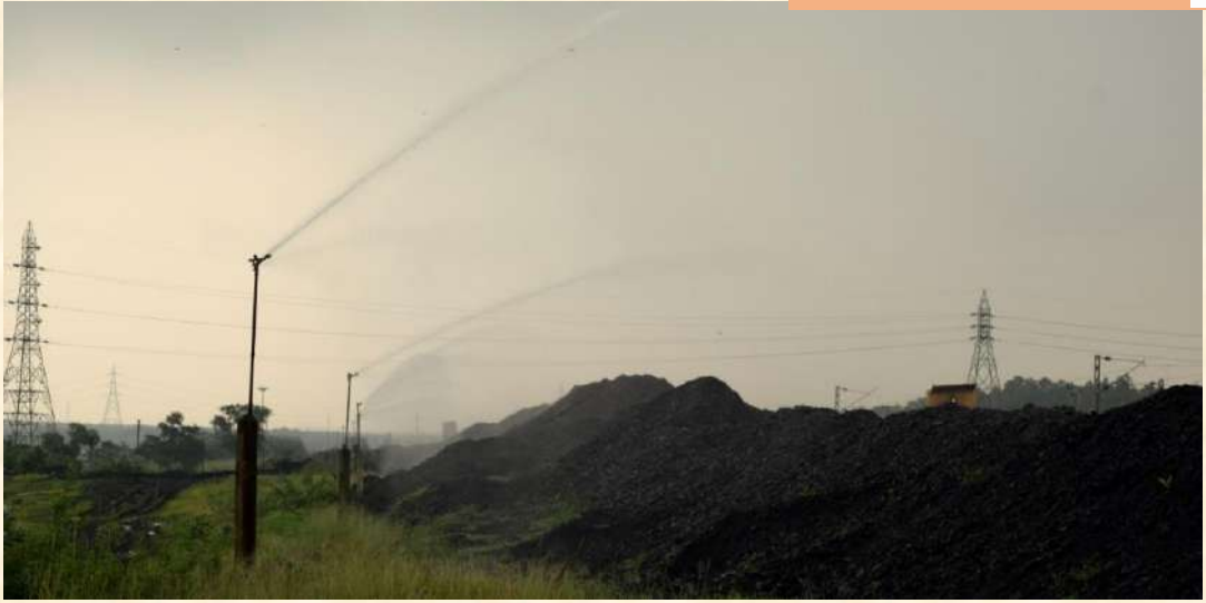
Fig. 46 - Fixed Sprinkler in Belpahad OC, MCL
