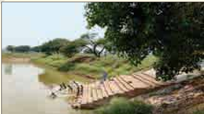
Image 3 : Construction and development of Pond for conservation of rain water at Gondwali Gram Panchayat.
