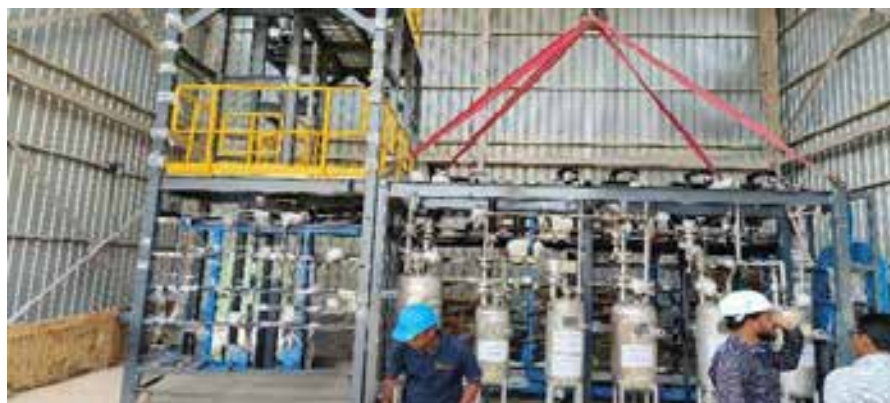
► Scaling up the conversion of CO 2 to Methanol and other value added chemicals
