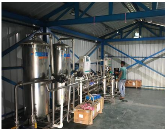
Fig. 51 - Mine Water to Drinking Water-Coal Neer in WCL
