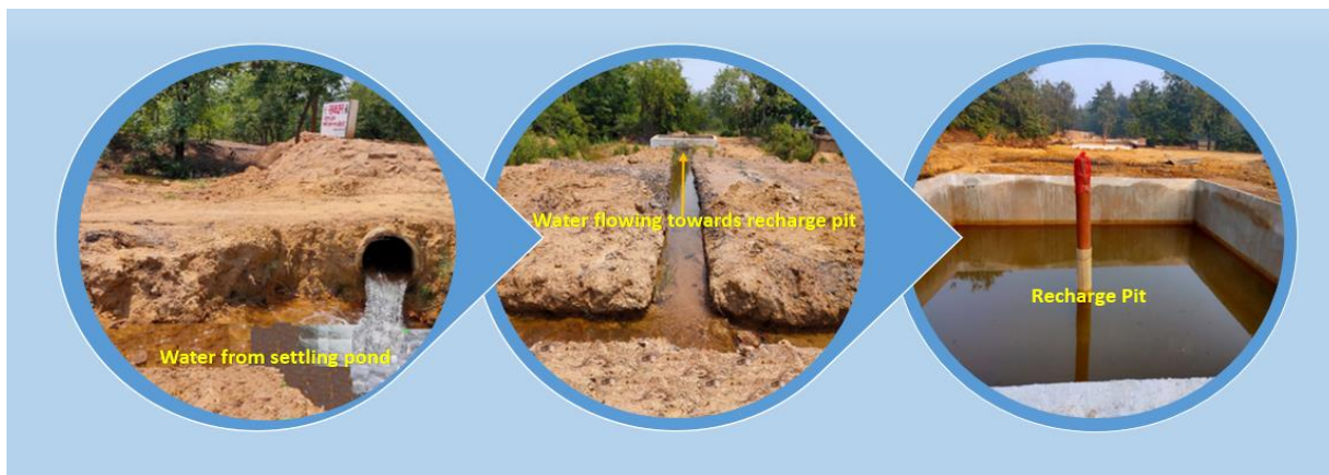
Fig. 55 - Ground Water Recharge Station in Samaleswari OCP, MCL
