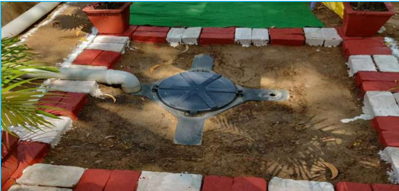
Rain Water Harvesting
