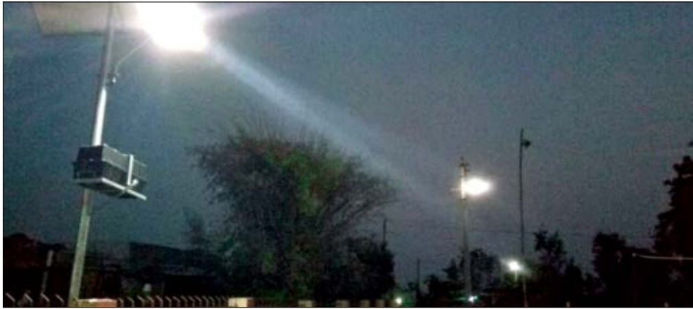
Energy Conserving LED Lights being installed by CMPDI, RI-IV in Nagpur, Maharashtra
