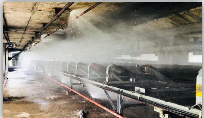
Fig. - Fixed sprinklers along belt conveyor
