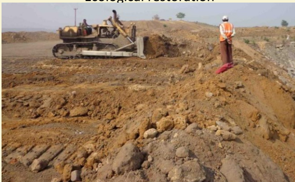
OB dump at Gokul Park, NT-St project, Lodna Area before Eco-cultural restoration
