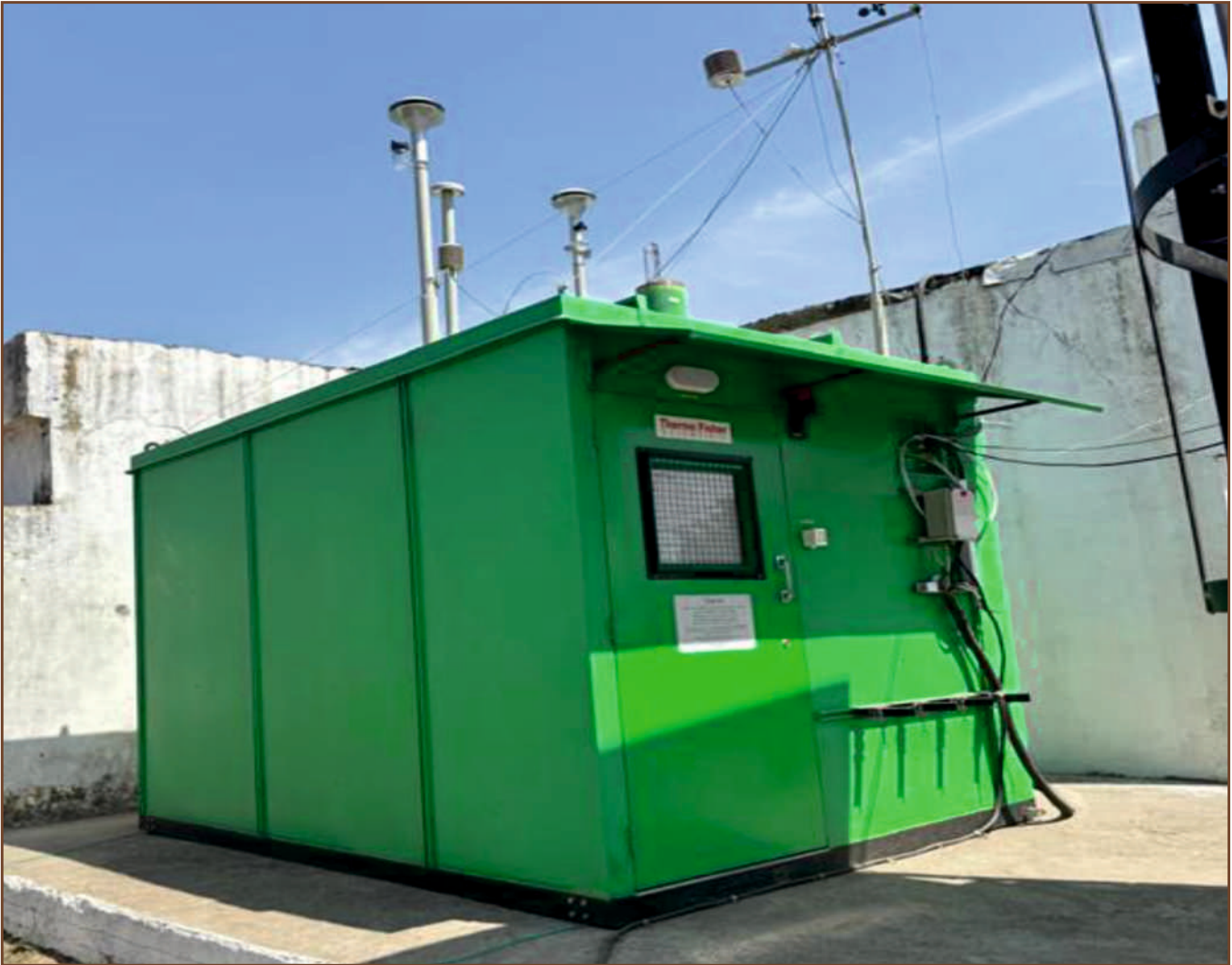
CAAQMS installed at VTC, Silewara UG Mine, Nagpur Area
