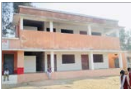
Construction of additional room with verandah in school at Bhakta village, Anuppur, MP near Baherabandh mine, Hasdeo Area
