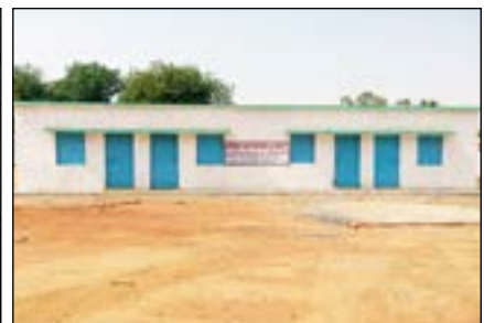
Construction of 04 Rooms at Government Girls High School Building at ward No. 09 of Bhatgaon
