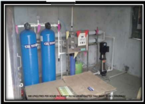
R.O Plant at Rehta Village
